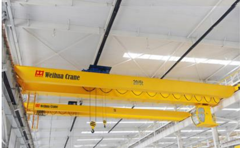
double girder bridge crane
